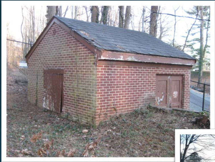
Royal Pump Station - 1920
