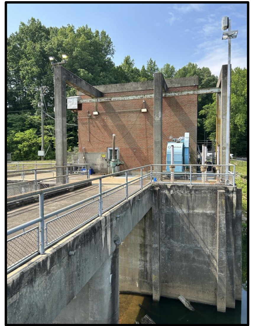
South Rivanna Raw Water Pump Station
