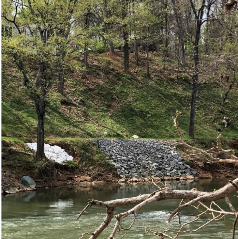
This area near Darden Towe Park required emergency repairs with riprap when erosion exposed utility lines in 2019
